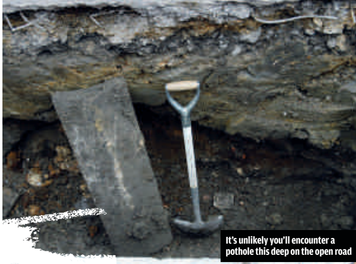
The road surface can break down around drains and manhole covers
